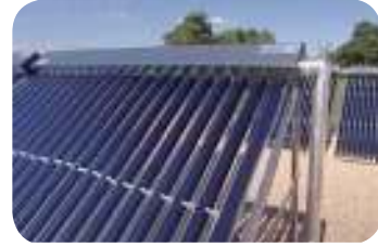
6. Solar panels producing heat
