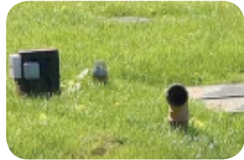
8. A self-contained sewer system
